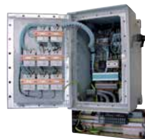
Ex d Panelboard with 8 Branch Circuit Breakers Coupled with Ex e Polyester Junction Box
